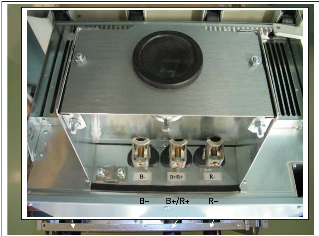
Figure 6-22. DC and brake resistor terminals on FR9; DC terminals marked with B- and B+, brake resistor terminals marked with R+ and R-
