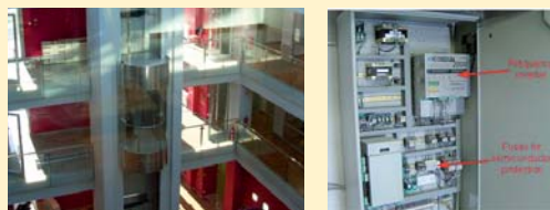
Frequency inverter for 3 phase AC motor (lift-elevator)
